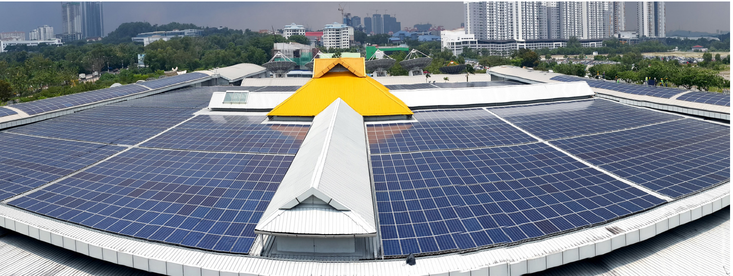
We installed more than 4,700 solar panels at Astro headquarters with the ability to generate 1.8 million kWh of electricity per annum
